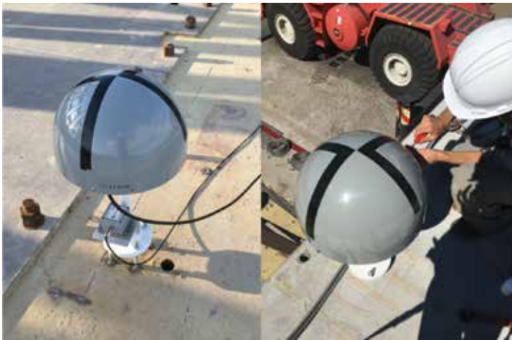
Figure 6. Installation of seismogeodetic instrumentation on a structure at the NHERI@UCSD Large High Performance Outdoor Shake Table. (Left) GPS antenna and SIO MEMS accelerometer on the shake table platen. (Right) On roof of the structure. The black tape on the antenna covers serves as targets for georeferencing UAV images of the structure. We use these earthquake simulations to test real-time data collection and earthquake detection algorithms.
